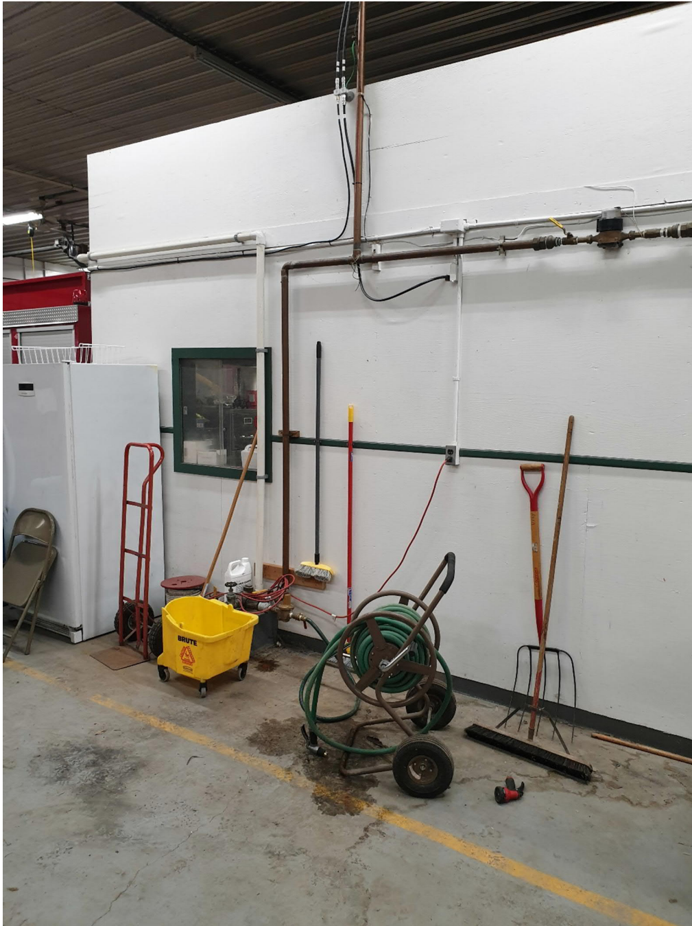
Existing meter location on domestic line in Fire Station. Proposed location for new meter.
