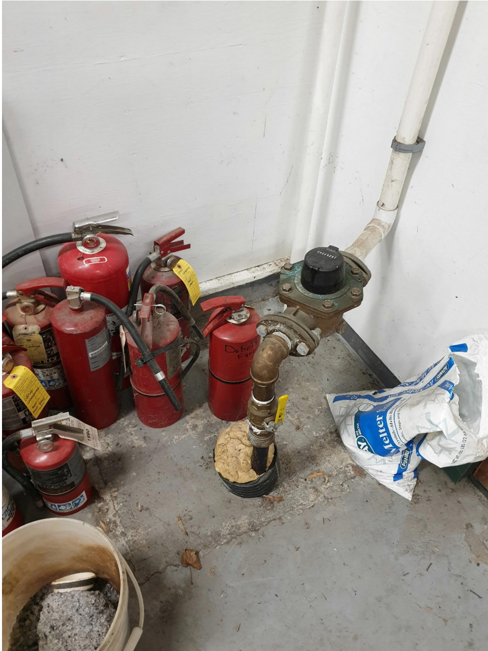
Existing meter location on line to fill trucks in Fire Station. Proposed location for new meter.
