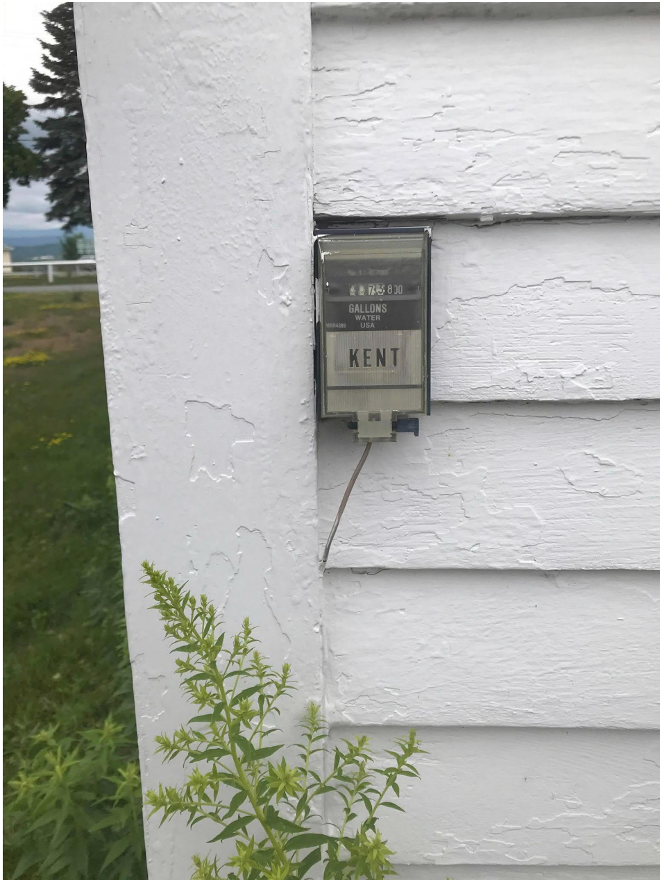
Existing meter read-out location for Church.
