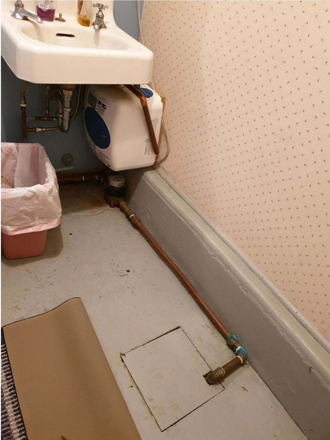
Existing meter location on domestic line in Church. Proposed location for new meter.
