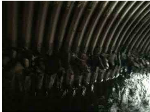
Severe section loss along the interior of pipe (bottom of pipe detached from top of pipe)
