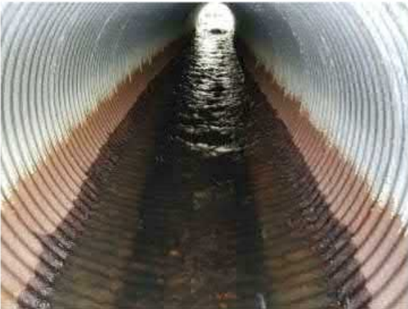
54-inch CMP with corrosion along the invert
